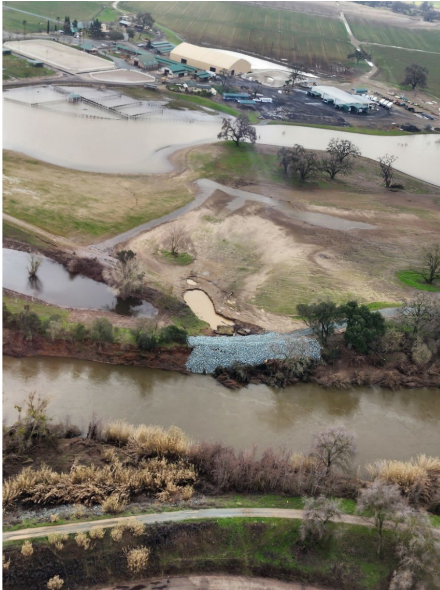
Figure 1 - impact of the storms on Reclamation District (RD) 800 levees and surrounding farmland.
